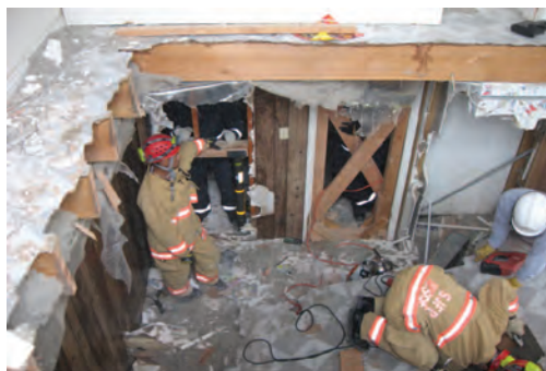
Figure 12- Rescue Crews train to respond to possible building damage caused by earthquakes.
