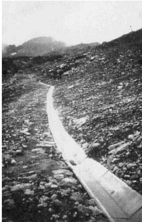
Surface water run off system by prefabricated channels
